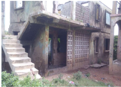
Plate 1. Building Destroyed by Flood. Source: Field Survey, 2018.
