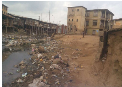
Plate 2: Partially collapsed building due to the flooding and waste clogging a stream.
